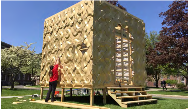
Figure 5: Crembil/Lokko “Golden Cube” Studio Installation at RPI School of Architecture, Troy NY.
