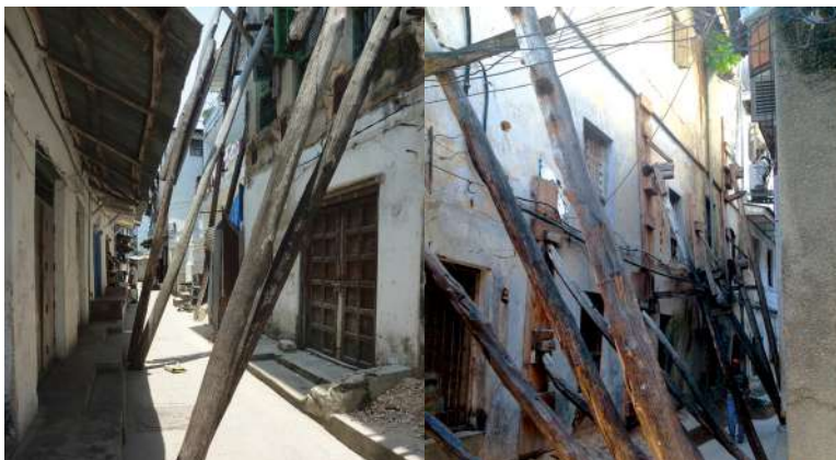
Fig.1 & 2: Alleys are sometimes almost completely blocked by intermediate support of instable buildings (Photos: Berend van der Lans)
